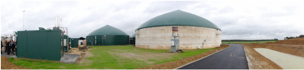
Figure 6: Biogas unit in Chaumes en Brie, France, owned by Bioénergie de la Brie Co. The plant produces biomethane and various products from agro food biowastes and manures. The biomethane is injected into the natural gas grid and feeds 5 cities located close to the unit.
