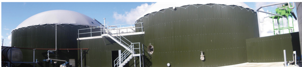
Figure 10: Biogas plant McDonnell Farms Limited. Primary Digester and first covered storage digester. David McDonnell milks 300 dairy cows in Limerick and also operates a free range poultry farm. In 2009/2010 he installed the most modern farm digester in Ireland which has a capacity of 250 kWh e . (Source: SEAI (Sustainable Energy Authority of Ireland) Anaerobic Digestion: A case study – McDonnell Farms Biogas Limited, Shanagolden, Co. Limerick))
