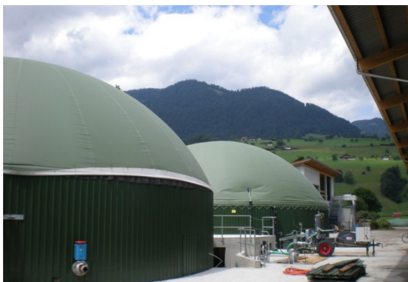
Figure 13: Biogas plant in Kägiswil, producing annually 1.5 GWh electricity and 1.7 GWh heat.
