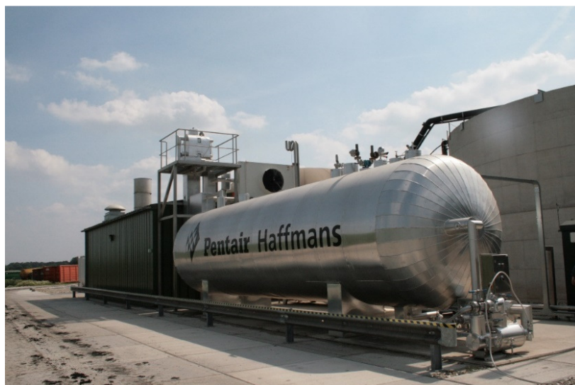
Figure 16: The biogas upgrading unit producing both biomethane and carbon dioxide at the Ecofuel biogas plant
